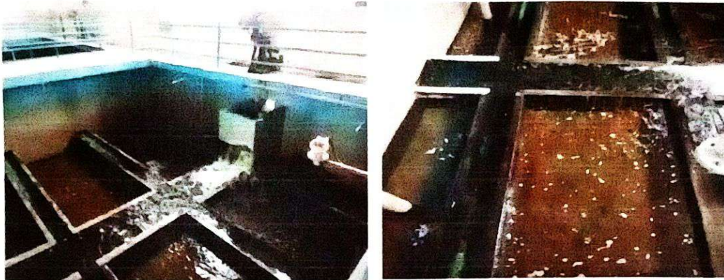
Fig. Rapid Sand Filtration Bed.
